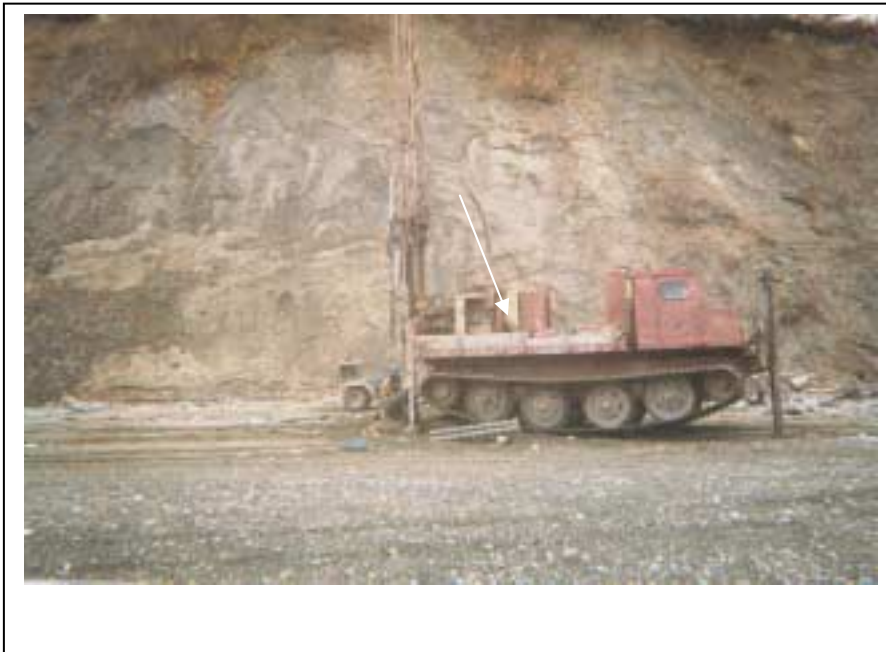
Photograph A-1: Nodwell CME-75 drill rig and east bluff at Boring A-13.
